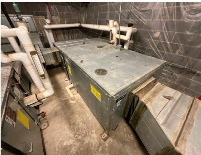
21 - TYPICAL AIR HANDLER
