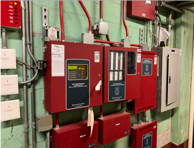
25 - FIRE ALARM PANELS
