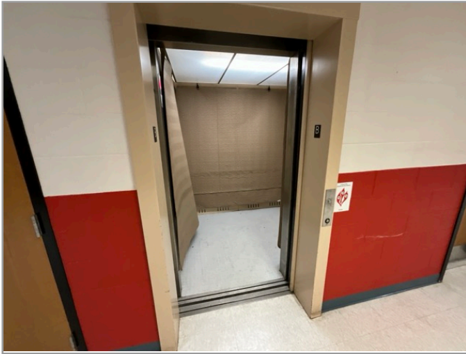
LOBBY LOOKING AT CABS (WITH DOORS OPEN)
