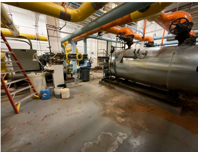
17 - MAIN BOILER ROOM
